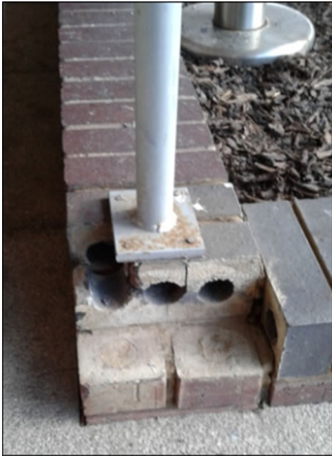
Fig. 5 Brickwork works loose which means the handrailing is non-compliant and potentially a hazard
