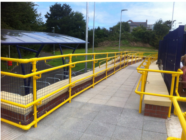
Fig. 6 Versatility of the fittings enabled long uprights to be included in the handrail systems at these potential fall risk locations
