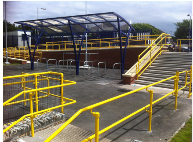
Fig. 3 Handrails constructed from tube and fittings along with 50 x 50 mm Weld Mesh Panels
